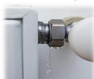
Leak detection in equipment and piping
