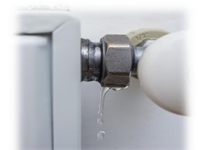
Leak detection in equipment and piping
